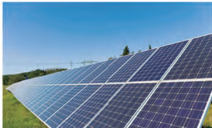
Yuzhou Peak Photovoltaic Power Station Project
